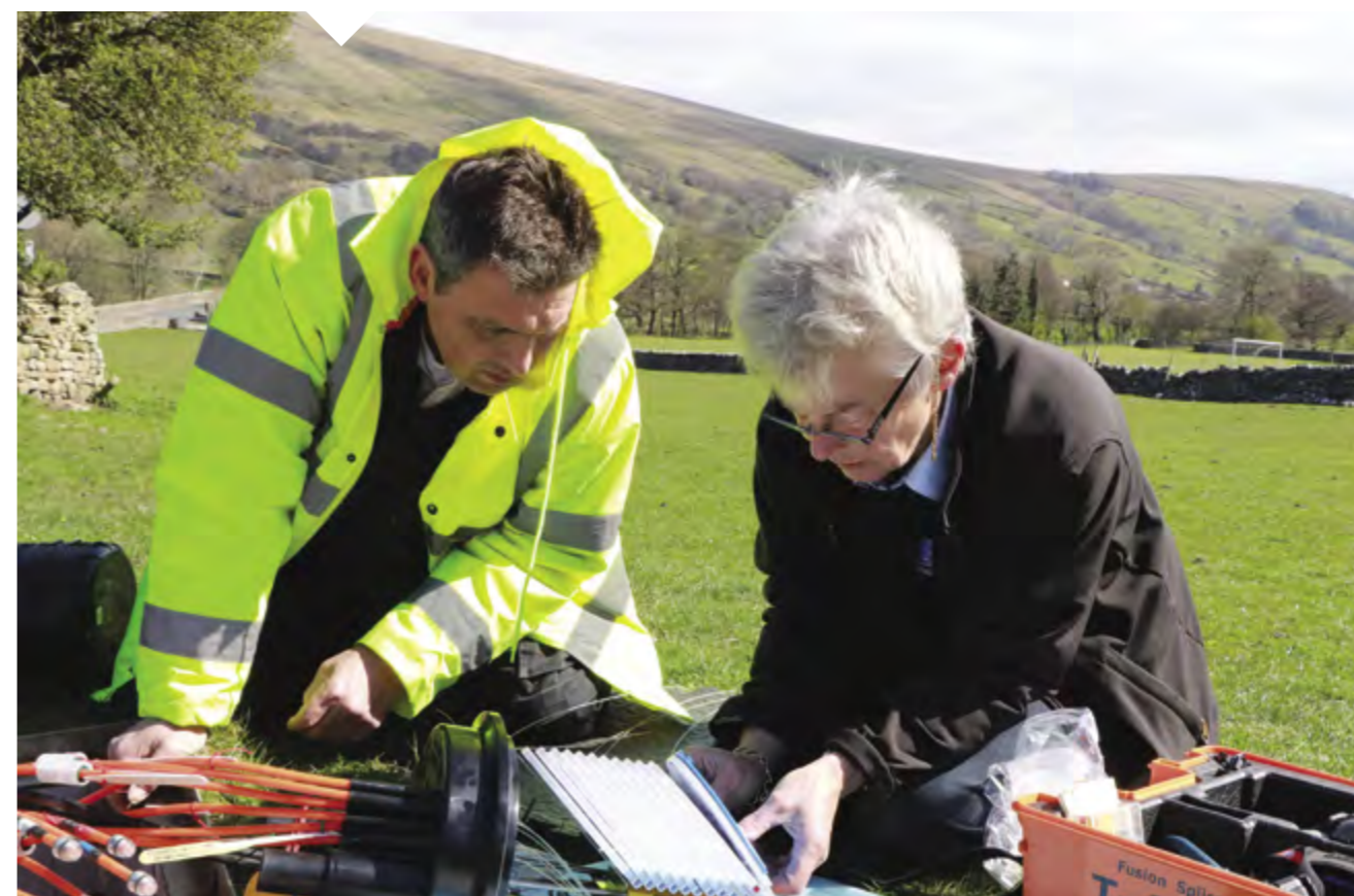
A B4RN volunteer showing another volunteer how to fuse fiber-optic cables in a rural field.
